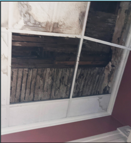
The ceiling in one of Franklin's rooms showing water damage.
