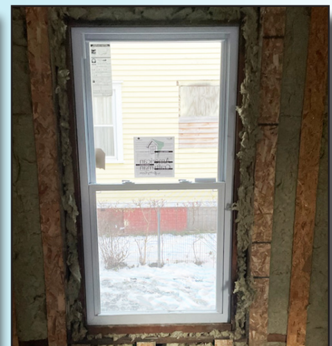
The room is gutted and an image shows one of the new energy-efficient windows.
