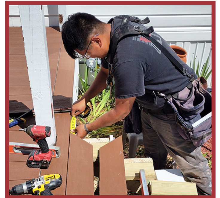
Edgar Herrera of Greater Springfield Habitat for Humanity's construction crew works on the new deck.
