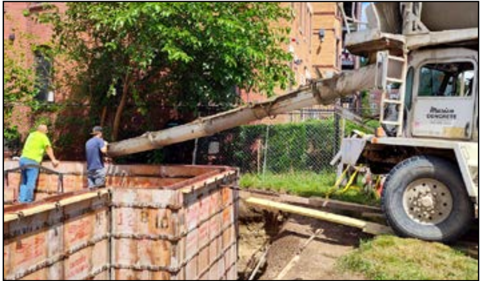
The cement walls of the foundation are poured at the build site of Greater Springfield Habitat for Humanity's newest home on Dwight Street in Springfield.
