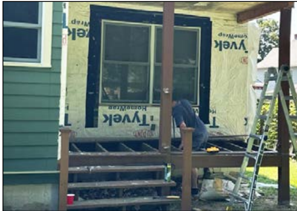
An employee from TNT General Contracting removes the deck from a property in Springfield to make room for a first-floor bedroom and bathroom addition.
