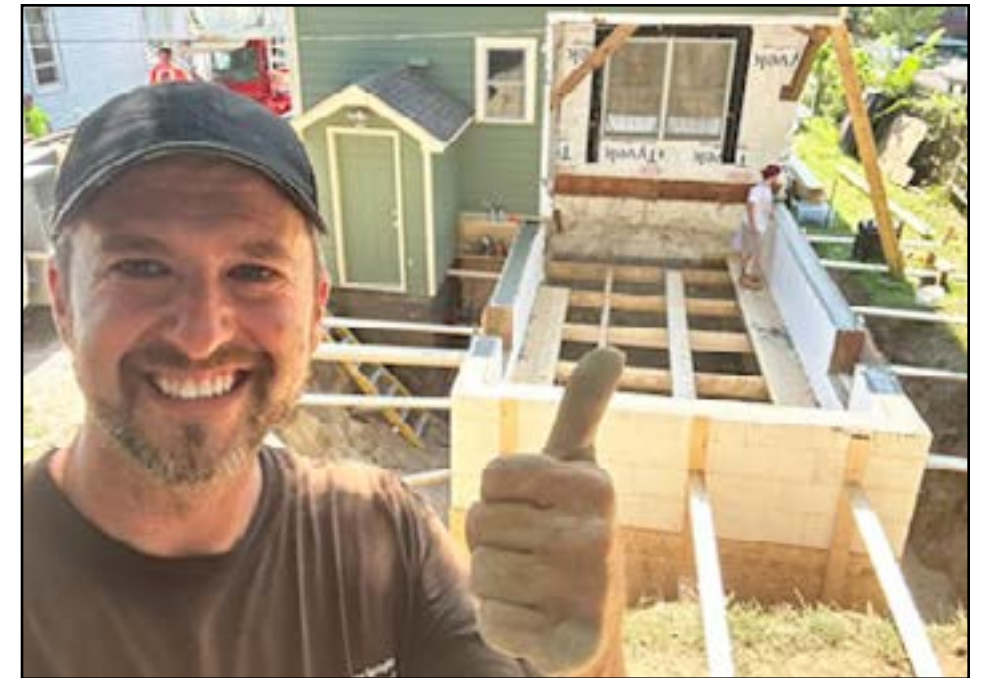
Walt Tomala, of TNT General Contracting, gives a thumbs-up as he shows the progress of the first-floor addition on Max's house. Instead of using wood frames, he is utilizing insulated concrete forms, which is more energy efficient, quieter, and less expensive than lumber.
