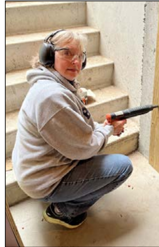
Cathy Faits uses a powder-actuated tool, also known as a Ramset gun, at the Bay Street build site in Springfield, to drive nails through wood into the concrete foundation to install the inner basement door below the bulkhead door.
