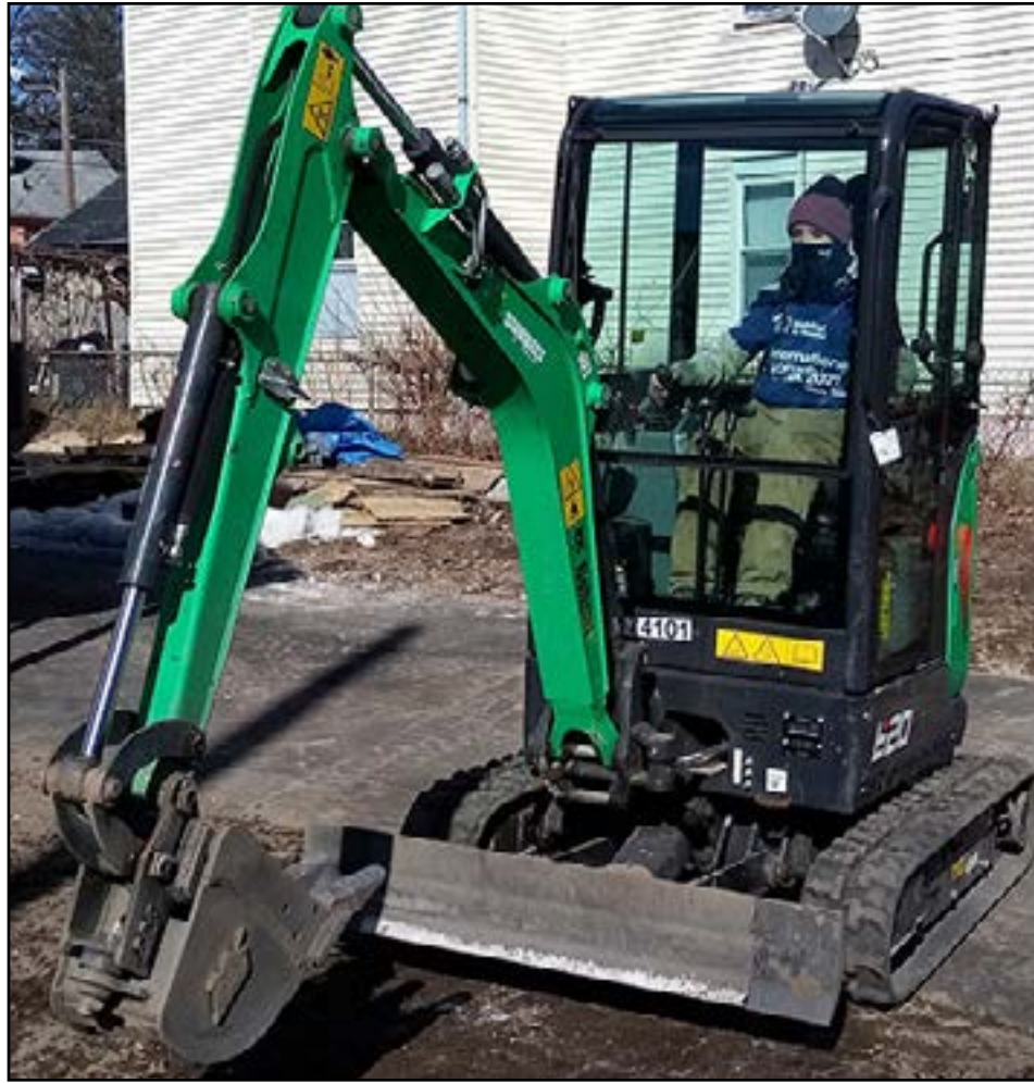
Amy Calandrella, a past Greater Springfield Habitat for Humanity (GSHFH) volunteer, operates an excavator at a previous build site for a new GSHFH home.
