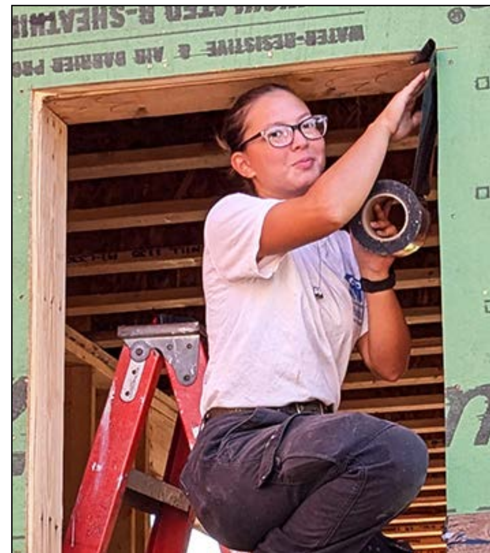
Violeta Melendez, a member of Greater Springfield Habitat for Humanity's construction crew, tapes a window cutout to prevent water from seeping underneath the sheathing.
