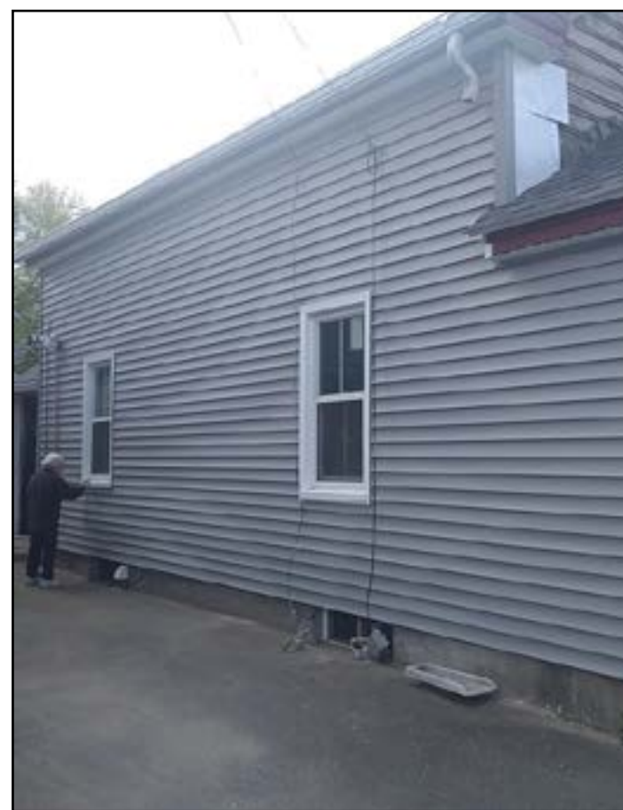
Phyllis dusts a new window sill on her Westfield house after siding went up.
