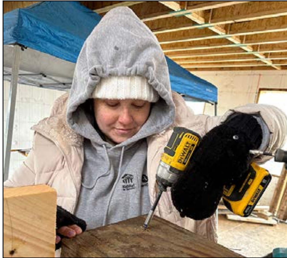
Samantha Majjad, Greater Springfield Habitat for Humanity's newest AmeriCorp volunteer, helps construct a staircase for the Chestnut Street, Holyoke, build site.
