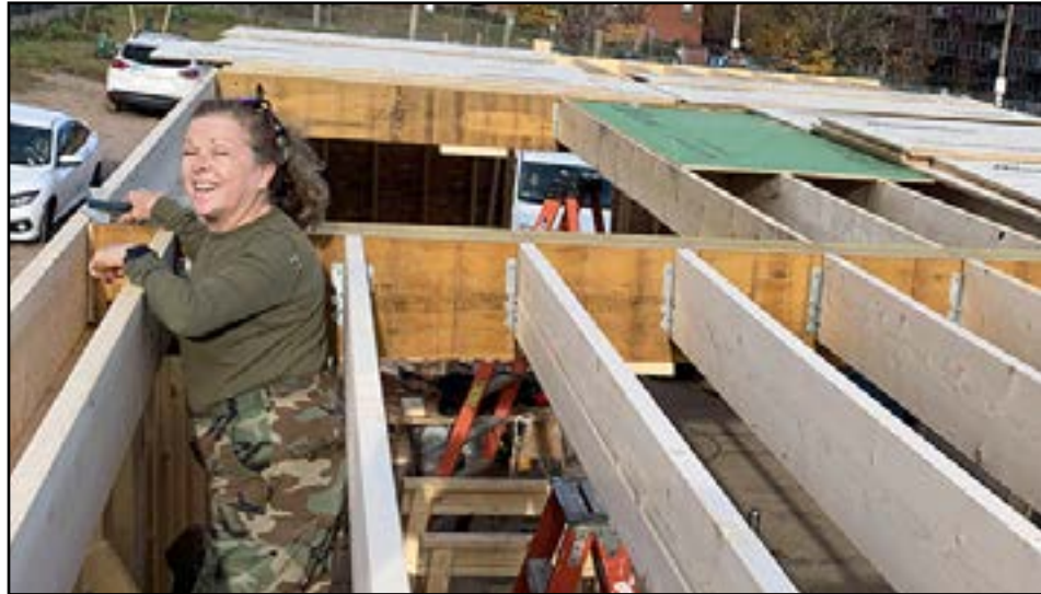
Lori Taylor, Greater Springfield Habitat for Humanity volunteer, helps build the second floor at a house in Holyoke.
