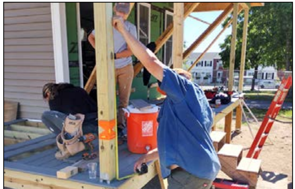
Greater Springfield Habitat for Humanity Construction crew, including carpenter Greg Garfield (front in blue) work to build a front porch on a house in Holyoke.
