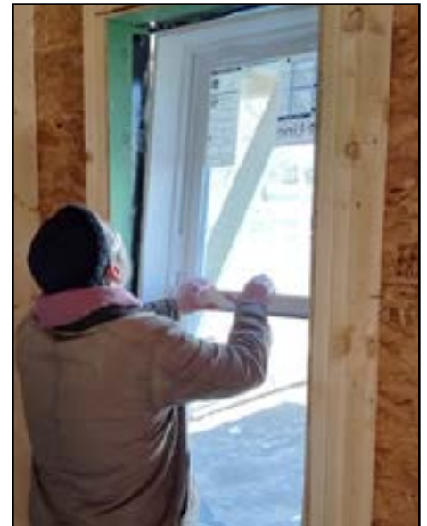
Community Works student Kel Spohn installs a window April 2 at a Holyoke build site.
