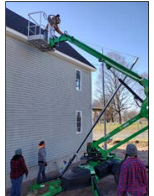
Top: A Community Works student taps the outside of the newly-installed window to put it in place.
