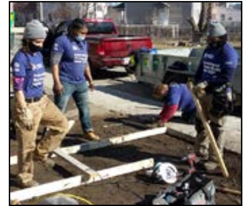
Tyeka Robinson second from left helps build a walkway during Greater Springfield Habitat for Humanity's Women Build event.
