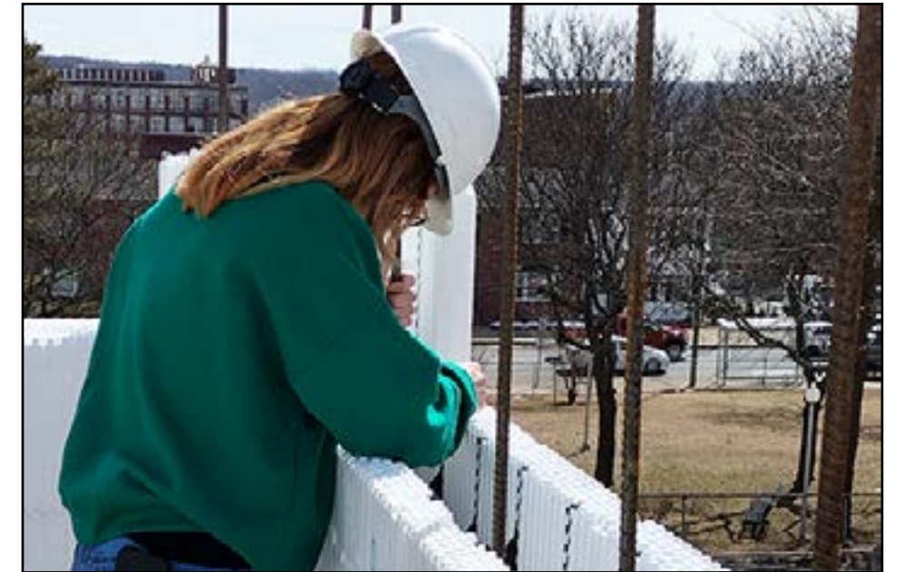
A student from Holyoke High School Dean Technical Campus places rebar between the IntegraSpec ICF foam blocks to give the concrete (after its poured) additional support.
