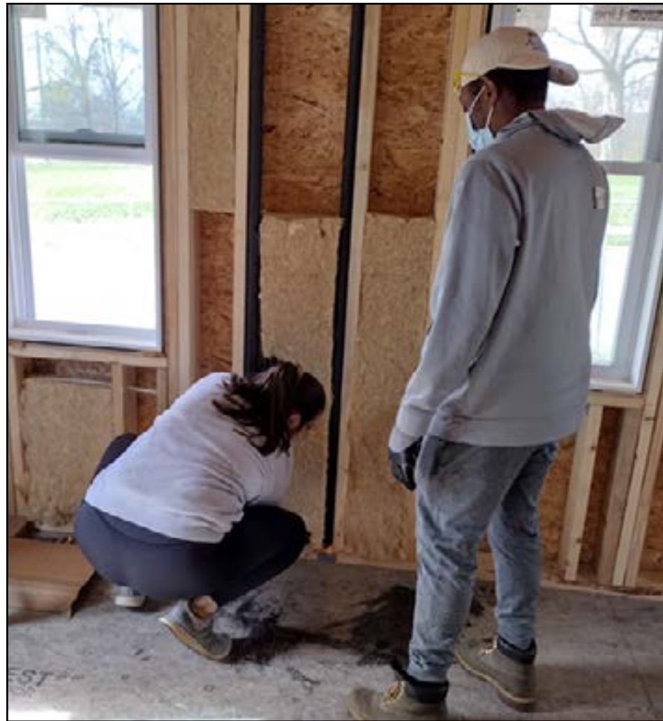
Students from Western New England University Pharmacy Degree program installed Hempitecture HempWool at our Jackson Street, Holyoke, build site in April 2022.
