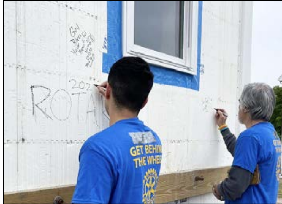
Greater Springfield Habitat for Humanity Volunteers from the Springfield Rotary Club autograph the insulated concrete foam frame of the Greater Springfield Habitat for Humanity's newest home at the Holyoke build site.
