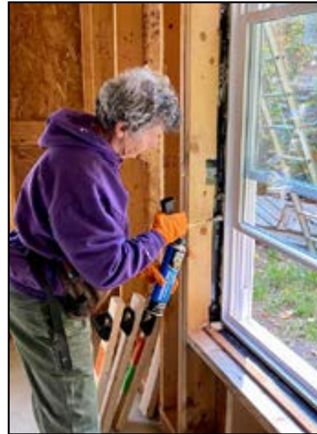
Pioneer Valley Habitat for Humanity Building tight and ventilating right is an important part of the “Pretty Good Home” design strategy. This picture shows a volunteer air sealing around a window.
