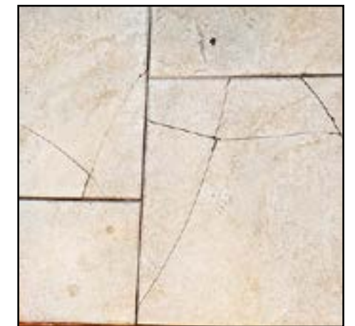
Above: the old, cracked ceramic tile. Top: the new laminate flooring in Tom and Dolores’s Indian Orchard home.
